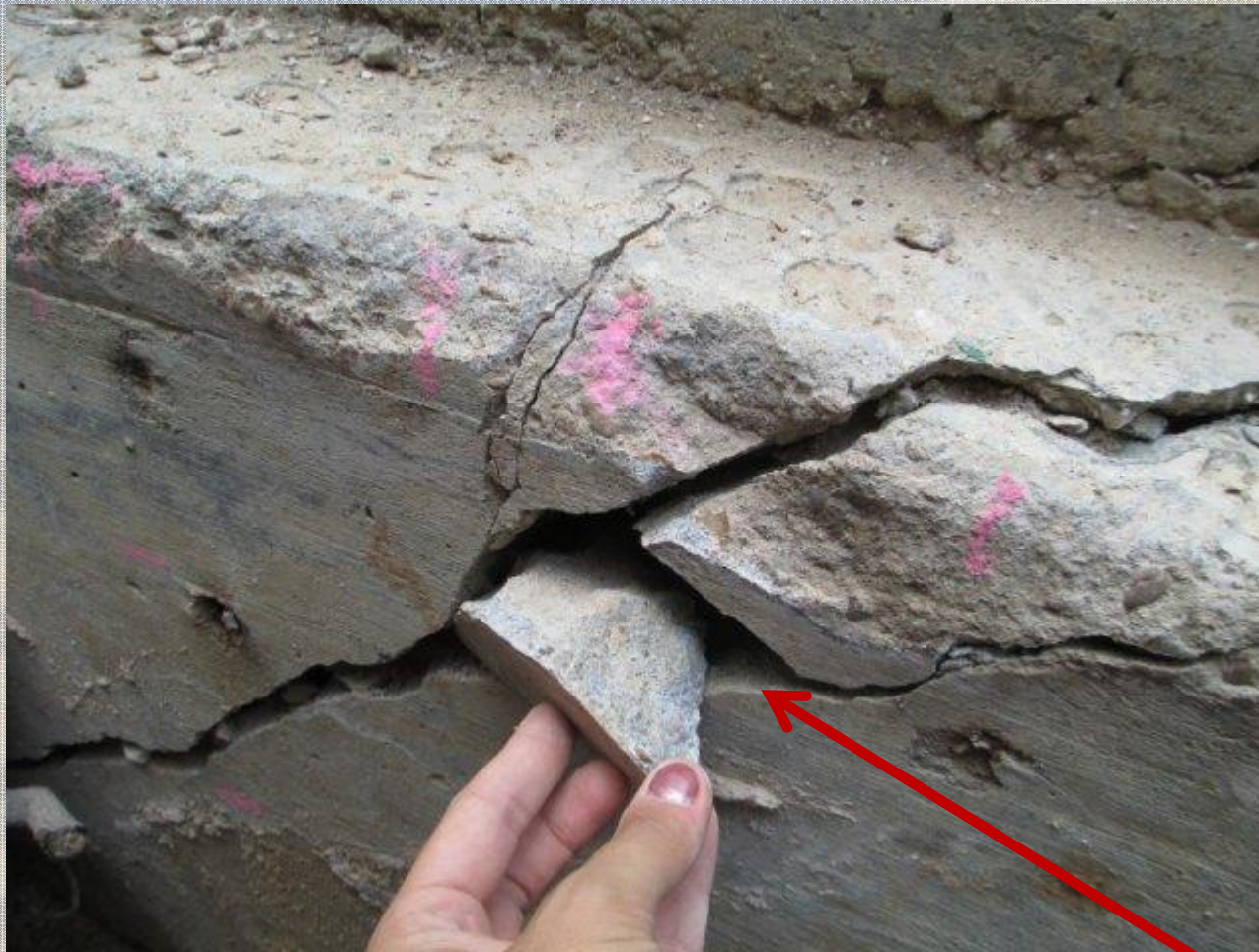
Another view of failed grade beam measured to have a 4 inch slope
